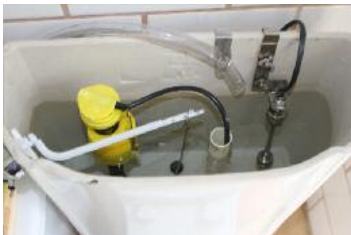
The clear plastic hose at the top of the toilet tank comes from the reservoir of cold shower water that is stored, rather than drained, from the shower.
